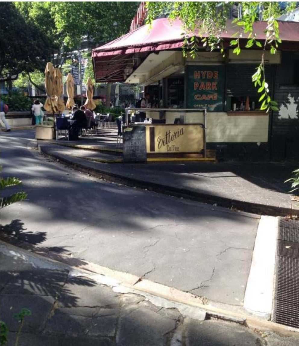
Image b) Museum Café – surrounding pavement areas damaged and uneven, creating accessibility issues
